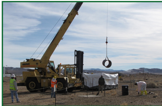
Debris removal and waste packaging activities at a contaminated site on the NNSS
